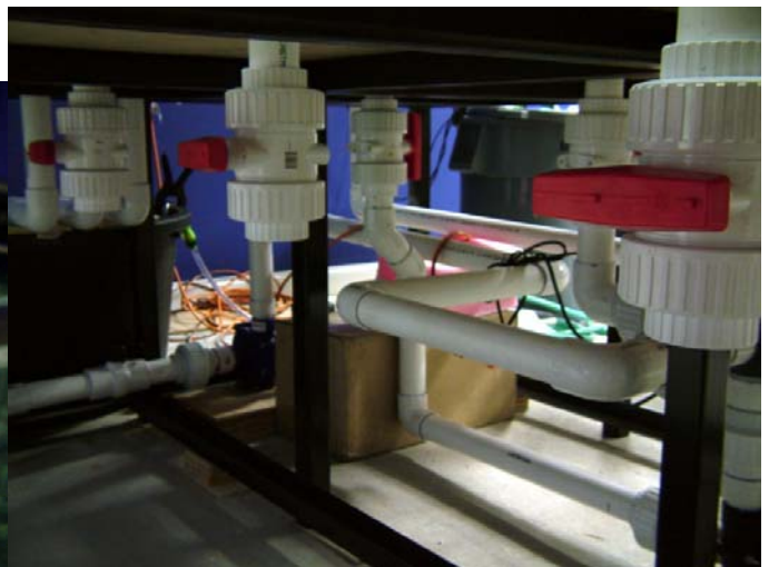
An Impressive Display of Plumbing Runs Underneath the Tank (above). Another View of the Tank Taken from A Different Angle Showing a Different Aspect of the Water Returns (below).
